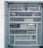
Modular Siemens controller with IEC 60'204 cabling
